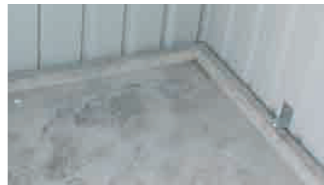
BUNDING TO MEET REQUIREMENTS FOR FIRE RESISTANT CHEMICAL SPILLAGE CONTAINMENT. NOMINAL CAPACITY - 120 LITRES PER BUND.
